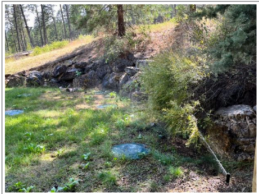
NEW SPRINKLERS AT WORK
